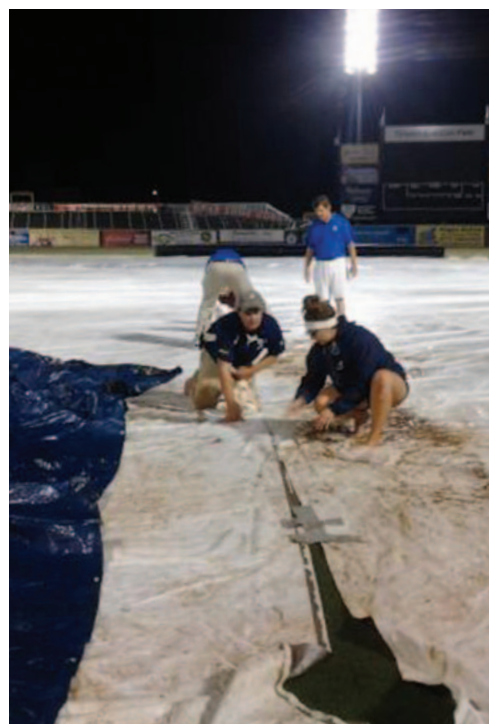
>> COREY RUSSELL leads his crew in repairing a torn tarp last summer in Myrtle Beach.
