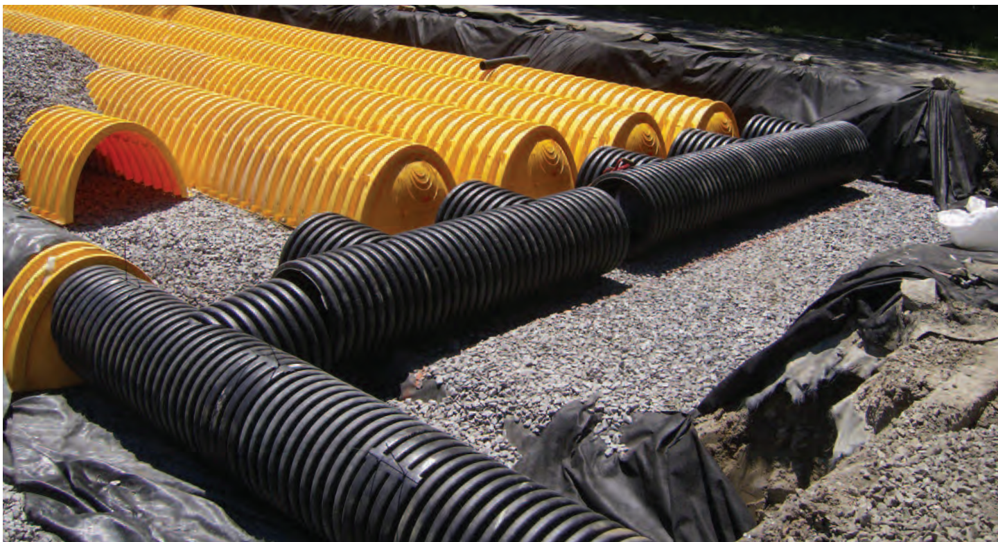
▲ THIS PHOTO , taken during construction of a sports field, shows piping at the entrance to the drainage chamber. Note the crushed rock beneath the pipe, which helps filter water vertically. All photos courtesy of Stantec, Boston, MA
