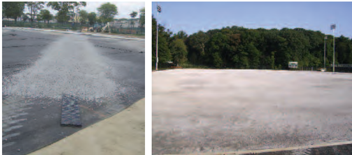
▲ LEFT: This cross-section shows the flat underdrain prior to installation in a field under construction. RIGHT: Sports field under construction showing the gravel drainage material.
