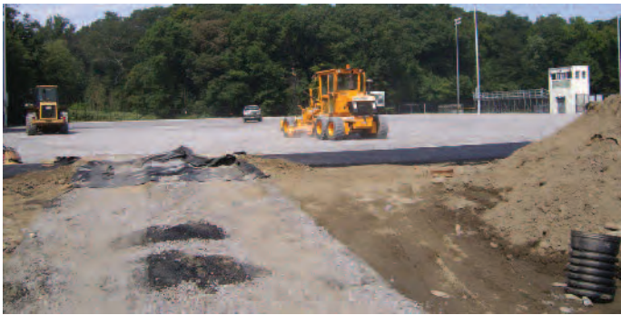
▲ A LAYER OF AGGREGATE is smoothed into place as part of the field construction process.
