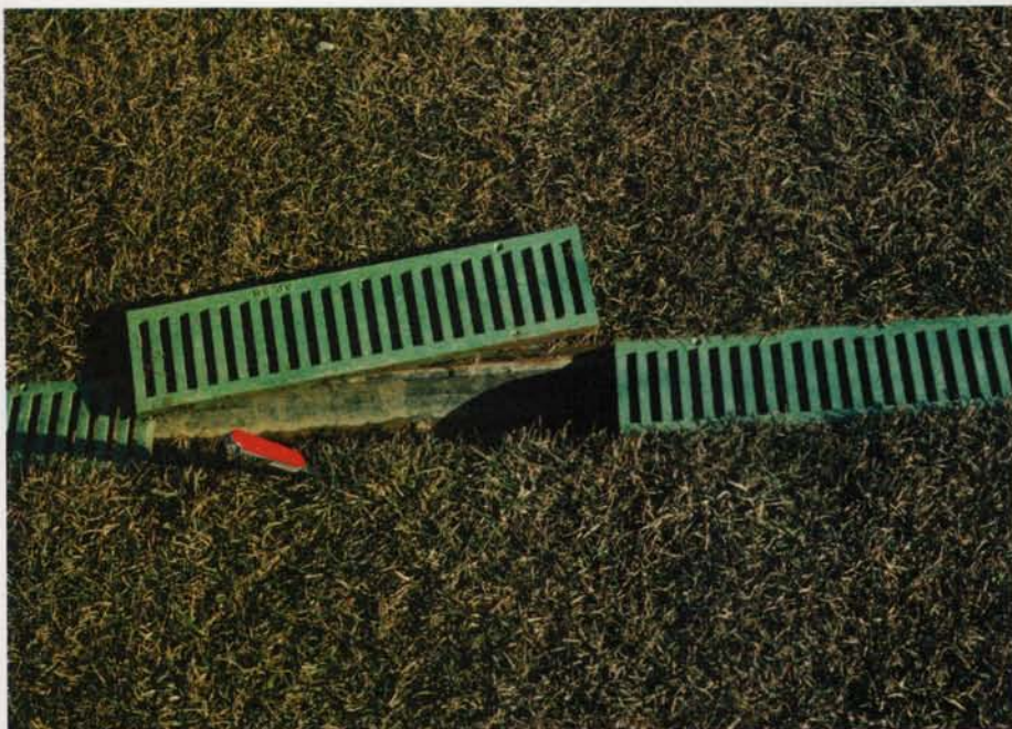
Close-up of split PVC and grate system at Beaver Stadium.
