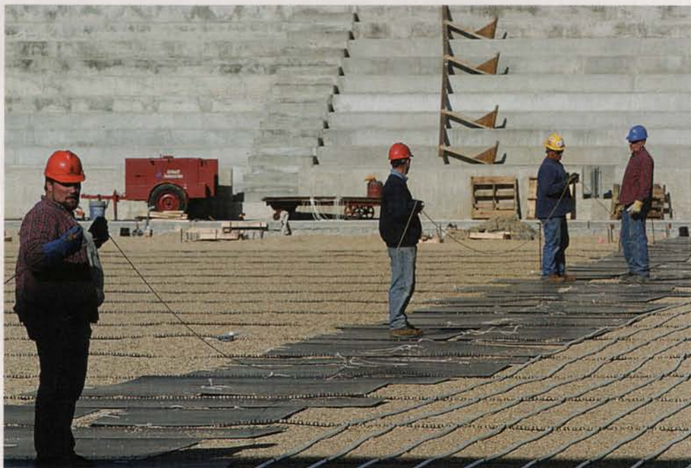
To prevent dimpling of surface with shoe prints, Althoff mechanics stood on sheets of Masonite while working on the field surface.
