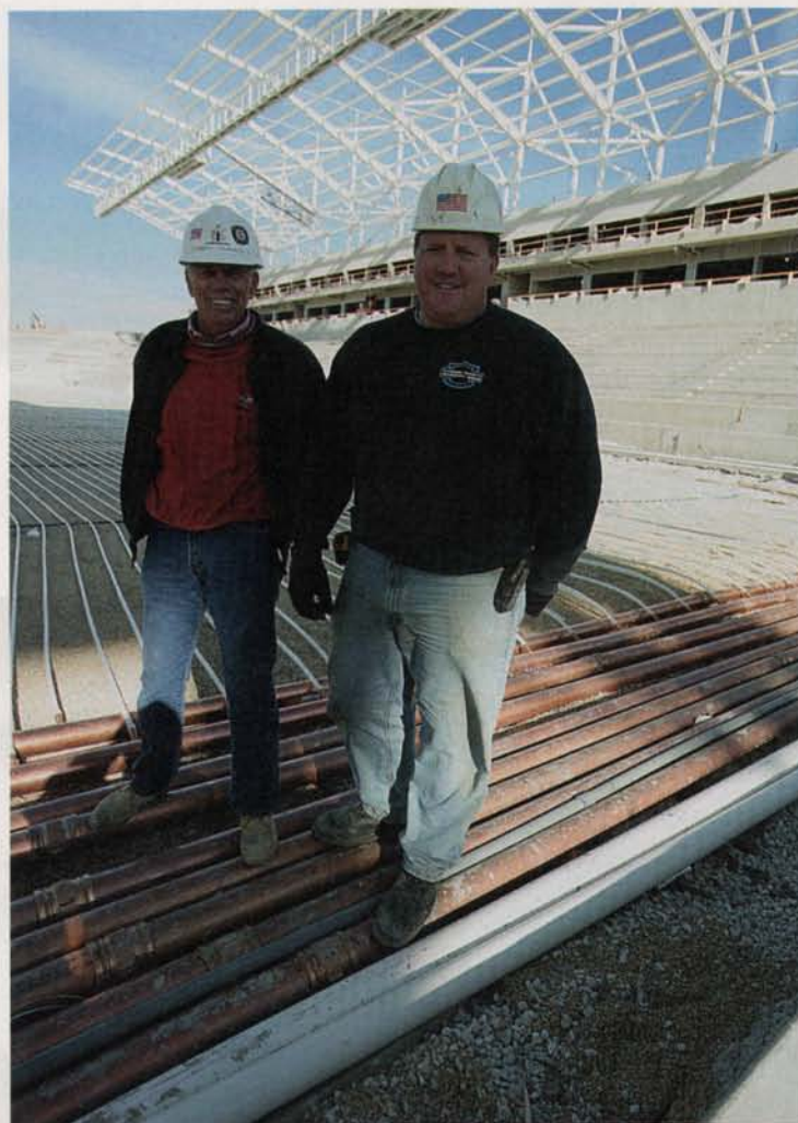
Project supervisor Chris Bennett (left), senior vice president at Althoff Industries, with John Lavin, shown in early November 2005, with the partially installed turf-conditioning system at the new Toyota Park in the background.
