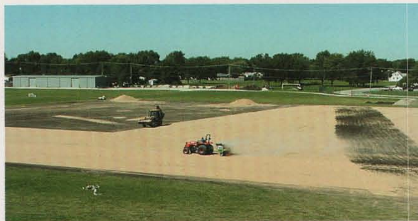
In preparation for the Chicago Bears' training camp, Olivet Nazarene University hustled last year to complete a $1.5 million renovation project, which included laying new sod, installing an underground irrigation system and adding TURFACE MVP to the fields.
