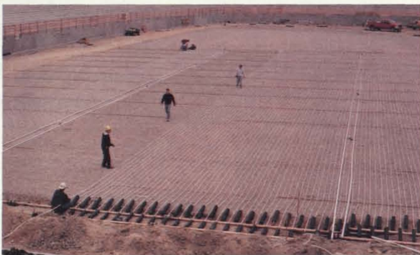
Each layer adds its own special tweak to the system, e.g., it's important to know what type of stone is to be used so its conductivity value can be accommodated.
