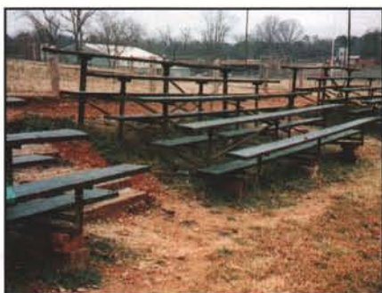
Create safe and presentable bleacher settings to prevent falls and mishaps. Courtesy: Floyd Perry
