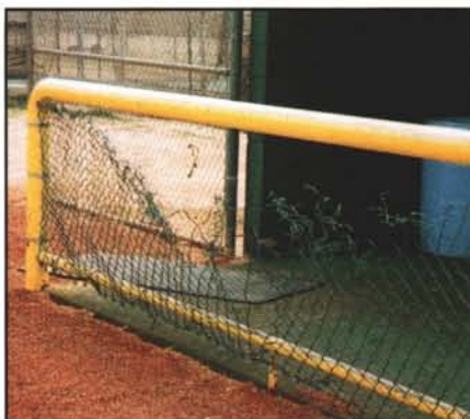
Repair damaged and potentially dangerous fencing. Courtesy: Floyd Perry
