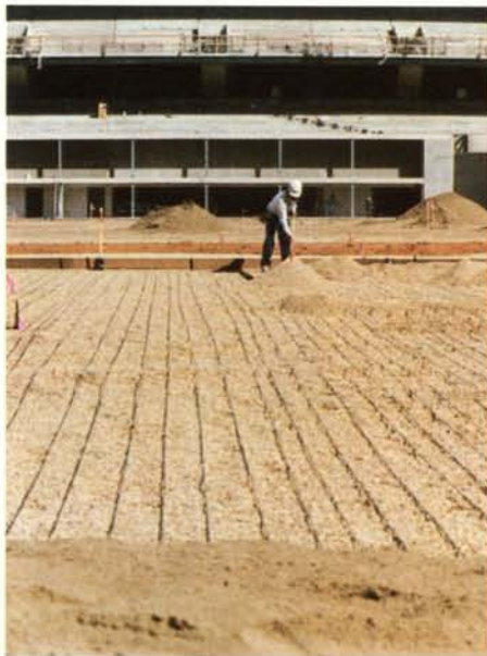
Coors Field in Denver, home of the Colorado Rockies, has 45 miles of underground heating cables installed in the rootzone. Photo courtesy: Randall & Blake, Inc.
