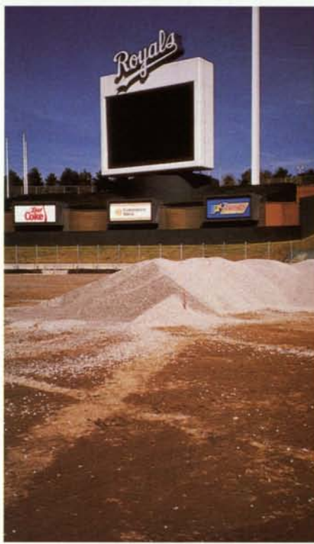
Pea gravel was spread four inches thick over the entire playing field except for the basepaths, home plate and the pitcher's mound. Photo courtesy: Vermeer Manufacturing Co.
