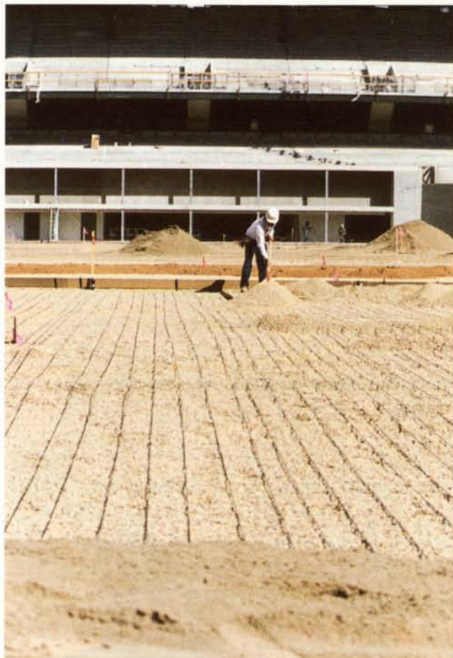
Forty-five miles of underground electric heating cables will keep the field at optimum temperatures. Photo courtesy: Randall & Blake, Inc.
