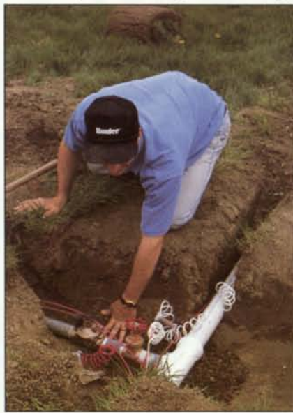
Undergraduate technology student Scott Gray wires a solenoid valve on a lateral line on the automated irrigation system.
