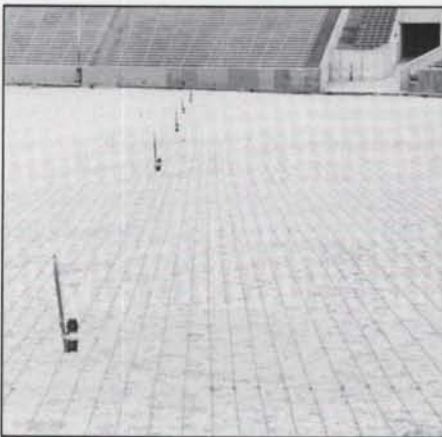
Electric heat cables and irrigation installed in pea gravel base.
