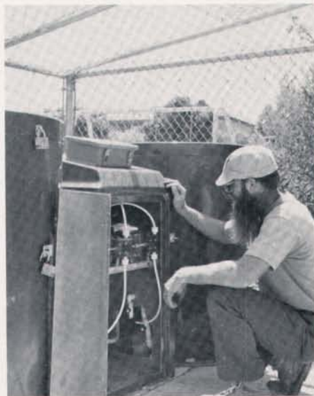
Nitrogen levels are adjustable to as low as 0.005 pounds per treatment during irrigation.
