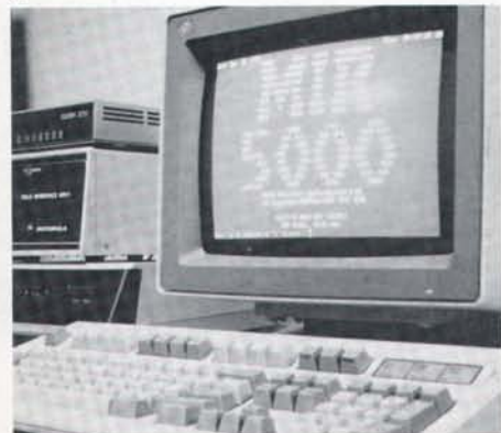
Central irrigation computer.
