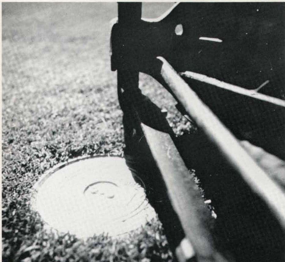
Sprinkler heads should be flush with the surface to avoid damage by maintenance equipment.
