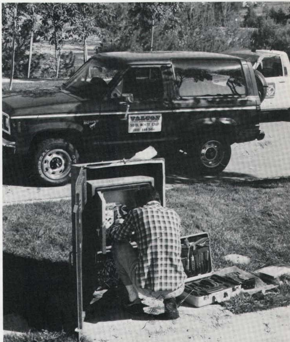
Technician checks resistance for each valve at controller.
