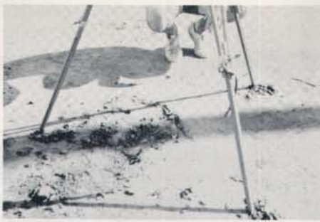
The transit's plumb bob must fall directly over the apex of home plate.
