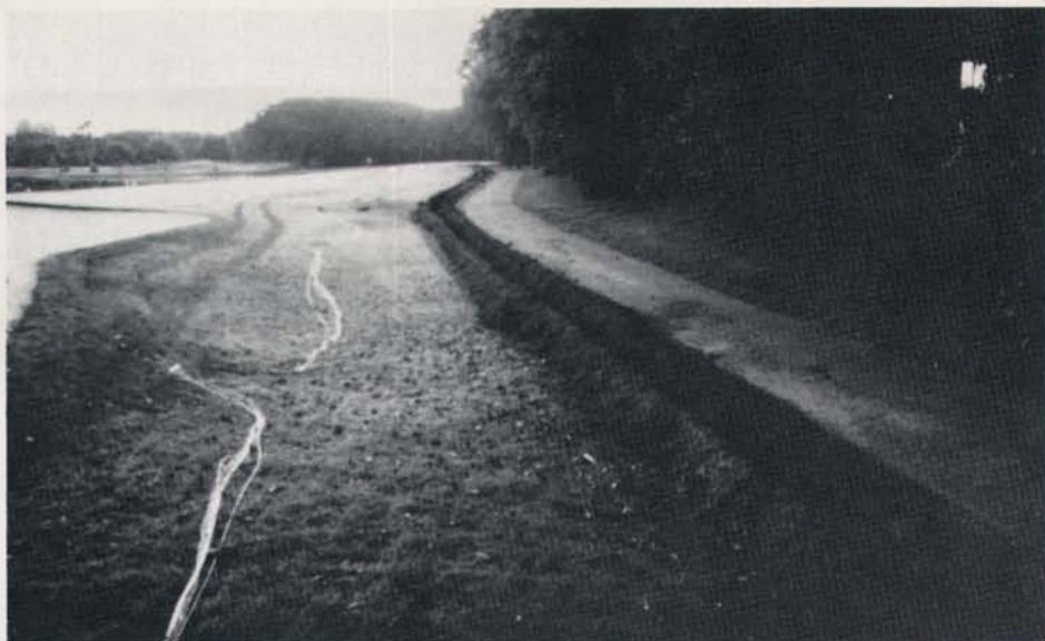
All wires, heads and controllers on the east course at Atlantis were replaced. The pipes on the newest of the three nines was left intact.
