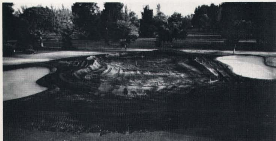
The greens on the east nine had to be rebuilt because muck soil used to construct them originally was causing severe drainage problems.
