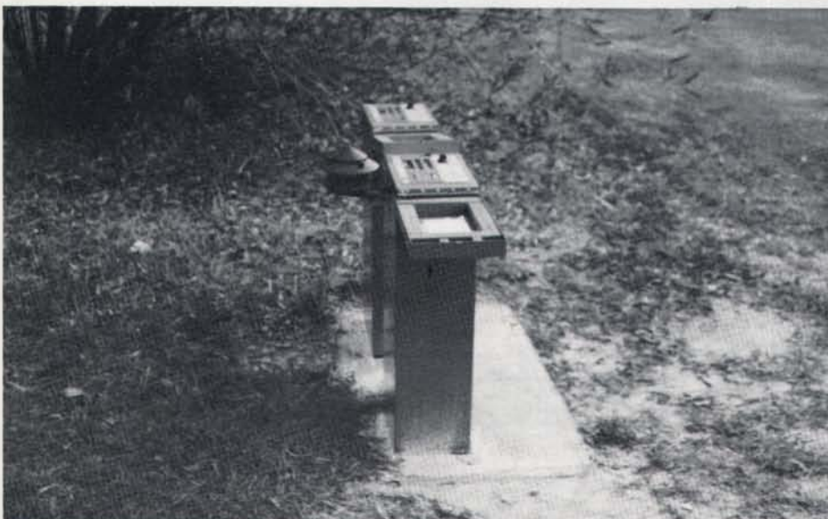
Irrigation programs are downloaded once each day to the satellites. The temperature monitor attached to these satellites feeds data to the central computer to determine daily ET.
