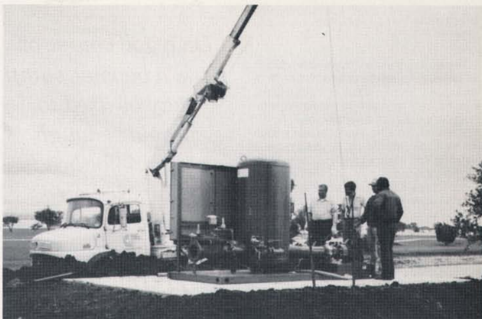
Prefabricated pump station being lowered on to pad at golf course. Photo courtesy: Carroll Childers.
