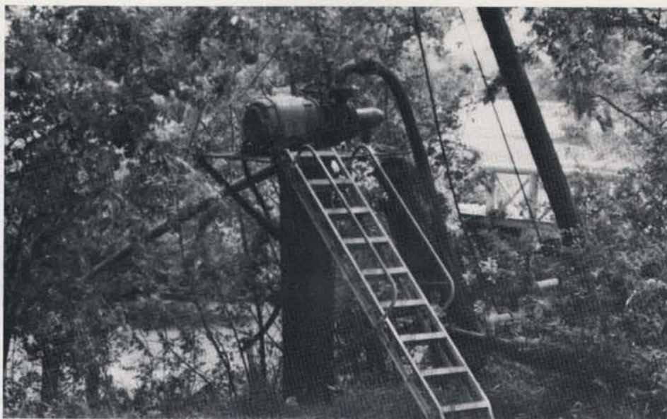
This pump, unprotected from weather and lacking pressure controls, is typical of older systems with poor energy efficiency.
