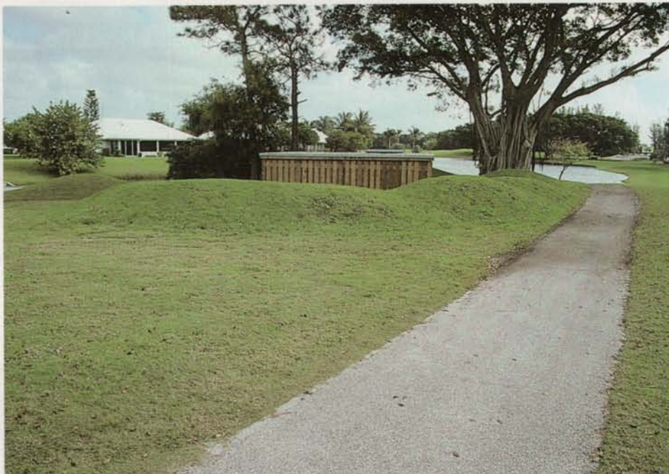
The new pump station at Atlantis is concealed in an attractive pump house nestled in a grove of trees. All pump components were hot-dipped galvanized to resist corrosion.
