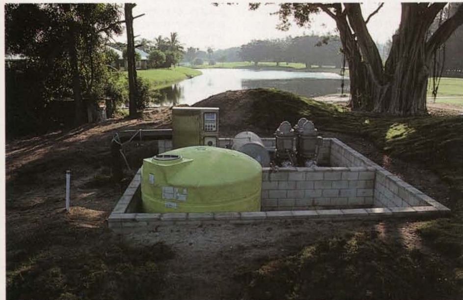
This single AquaTurf pump station replaced four separate pumps that were previously located at different locations on the 27-hole course.
