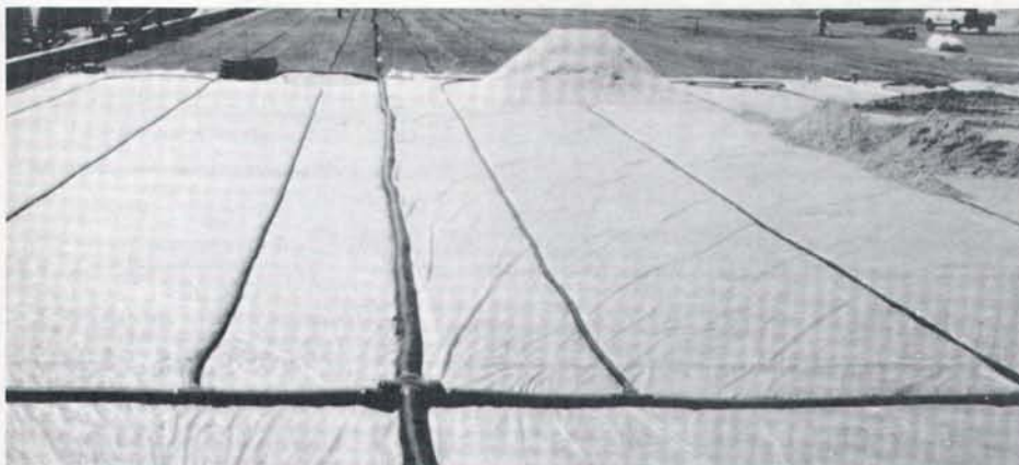
Drainage/subirrigation lines are set in trenches on top of the moisture barrier.
