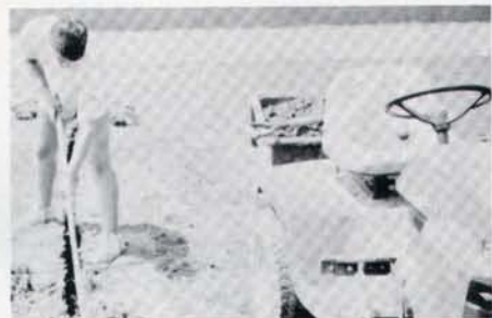
Turf Drain in the outfield was installed by the Texas A&M grounds crew.
