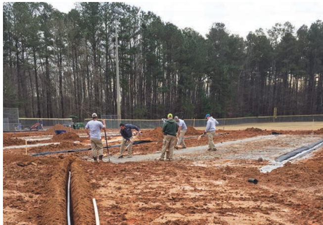
The construction process to build the sand-based infield on Bond Park field 5.
