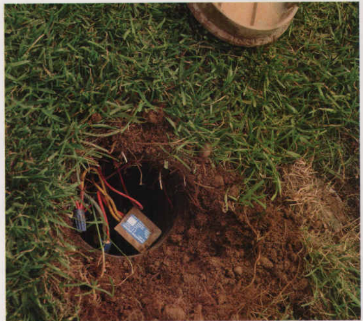
Underhill decoders are attached to every valve and irrigation programming is relayed to each valve over the two-wire system.
