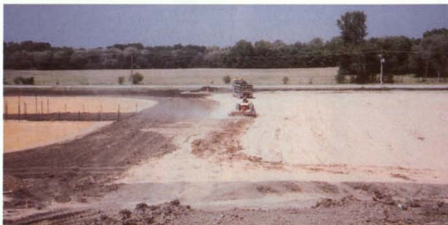
In the combination softball outfield and soccer field, calcined clay was incorporated into the soil to a depth of four to six inches.
