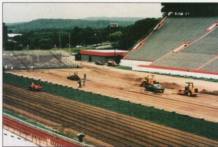
A layer of crushed gravel was laid as a sub-base and topped with 10 to 12 inches of a sand and peat mix.
