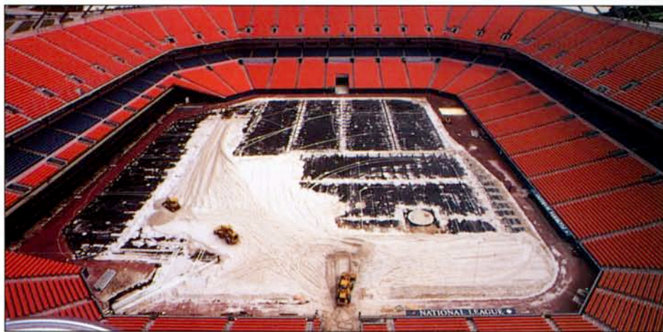
Joe Robbie Stadium undergoes sand profile distribution, covering drain lines and irrigation lines. Photos courtesy: The Motz Group and Deborah Gray Mitchell.
