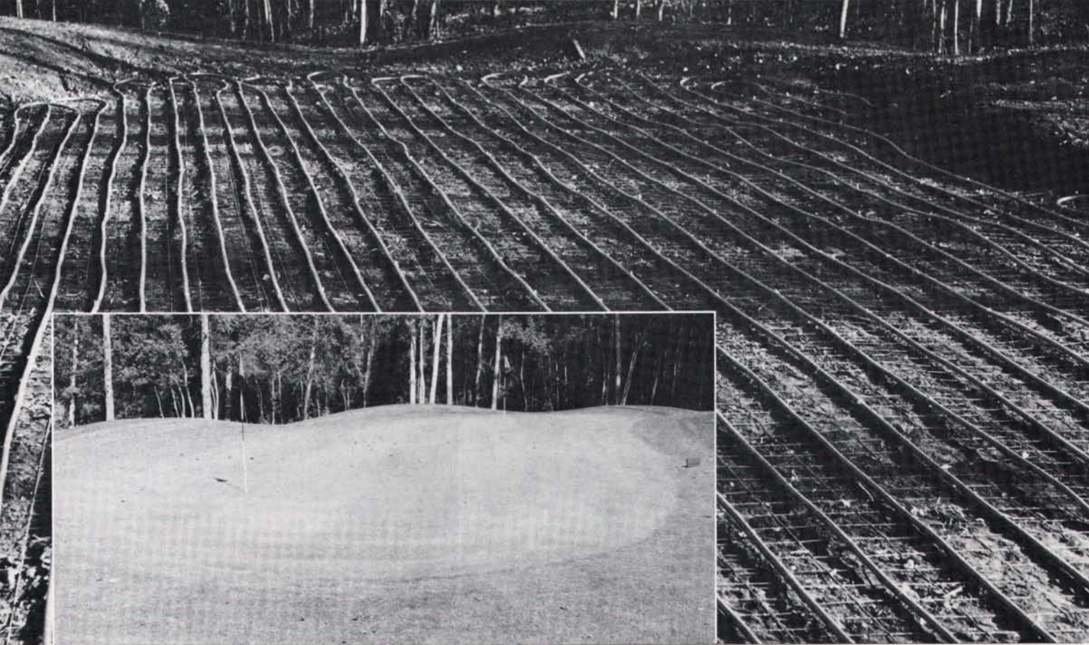
Cross-linked polyethylene tubing carries warm water/glycol mixture under practice green. Inset: Same green one year after heating system installation.
