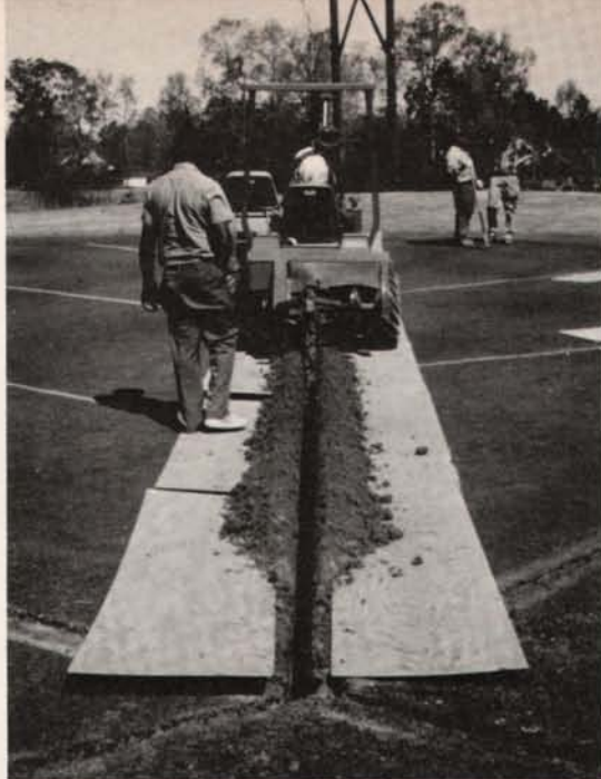
Installing bypass drainage in green at Shenandoah Country Club in Baton Rouge, LA. Photo courtesy: Turf Drainage Co. of America.
