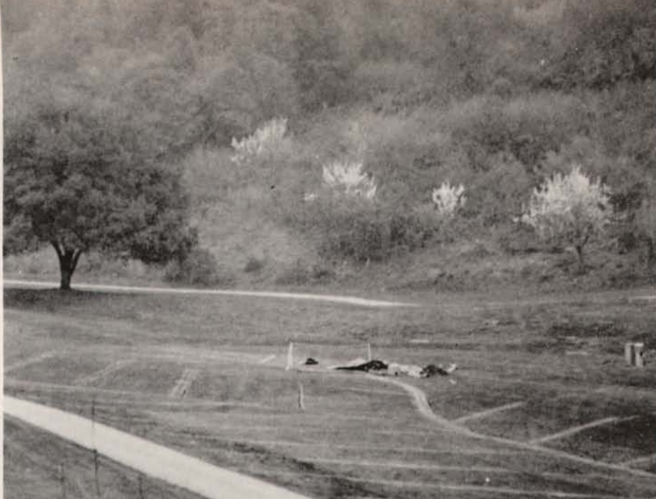
Herringbone pattern of bypass drainage installed at Saratoga Country Club in Saratoga, CA. Photo courtesy: Turf Drainage Co. of America.
