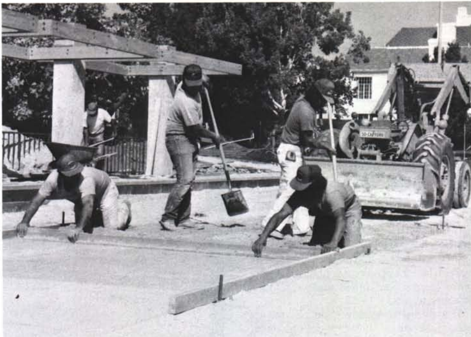
To come within a 1/16 inch tolerance on the greens at Roxbury Park, the crew from American Landscape Inc. installed the sand like they would concrete.
