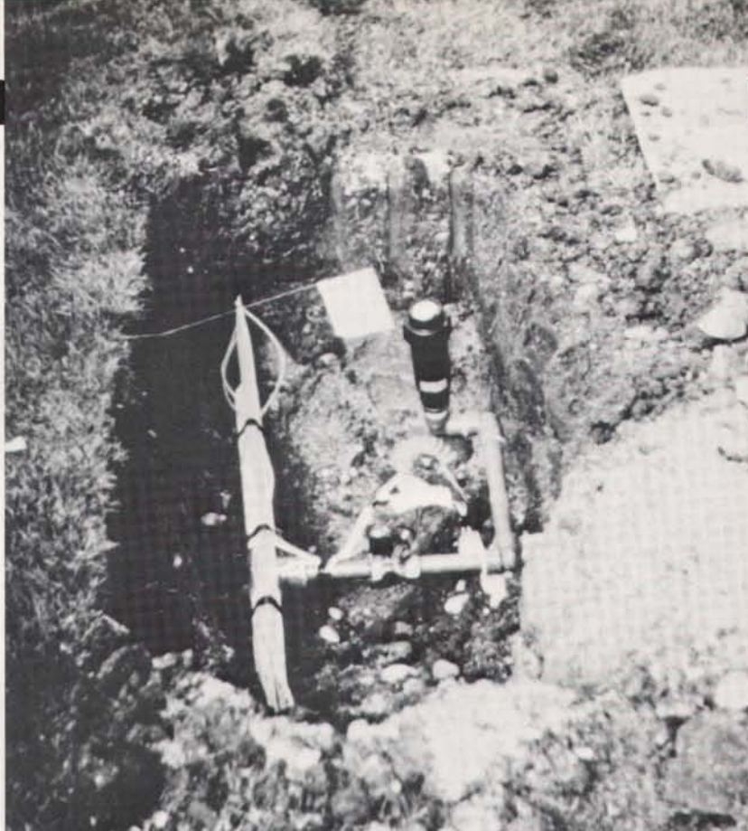
Surface damage was kept to a minimum while installing heads and valves since the field would be used by the Green Bay Packers in less than ten days.
