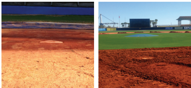
▲ Left: Leveling home plate with mound clay at Stone County High School, Wiggins, MS. Field maintained by head coach Hayden Cox. Right: Adding clay to the Pensacola Blue Wahoos Field, Pensacola, FL, where Ray Sayre is head groundskeeper.
