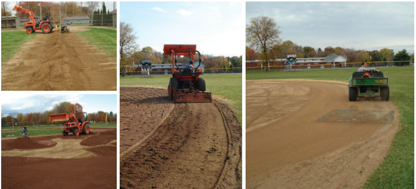
▲ Top Left: Excess skin soil is being removed from the base path to improve surface drainage. Bottom Left: A tractor is being used to spread the amendment evenly over the entire skinned area. Middle: The amendment is being rototilled into the existing skin soil at the recommended rate. Right: Notice the color is dull because the amendment is dusty from the tilling process.
