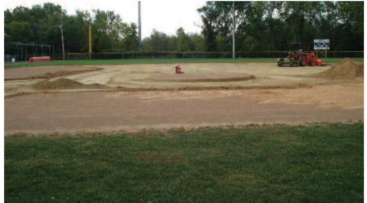
▲ After grading for surface runoff, 3 inches of skin soil is being removed in preparation for the new skin material.
