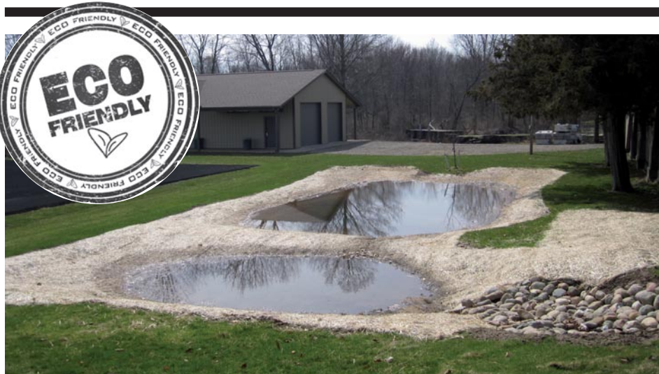
» A RAIN GARDEN designed to handle run-off from tennis courts, instead of directly into the river. An example of an Albion College's projects initiated and built to demonstrate future parking lot designs.
