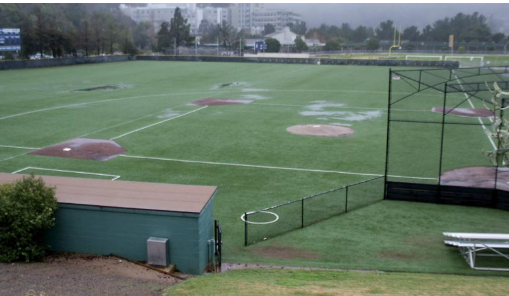
>> Above: POOR DRAINAGE of synthetic turf must be traced back to its source. It may be an easy fix (such as clean-outs that have become clogged with debris) or it may be something requiring extensive work. Photo courtesy of William E. Fee, Carducci Landscape Architects, San Francisco.
