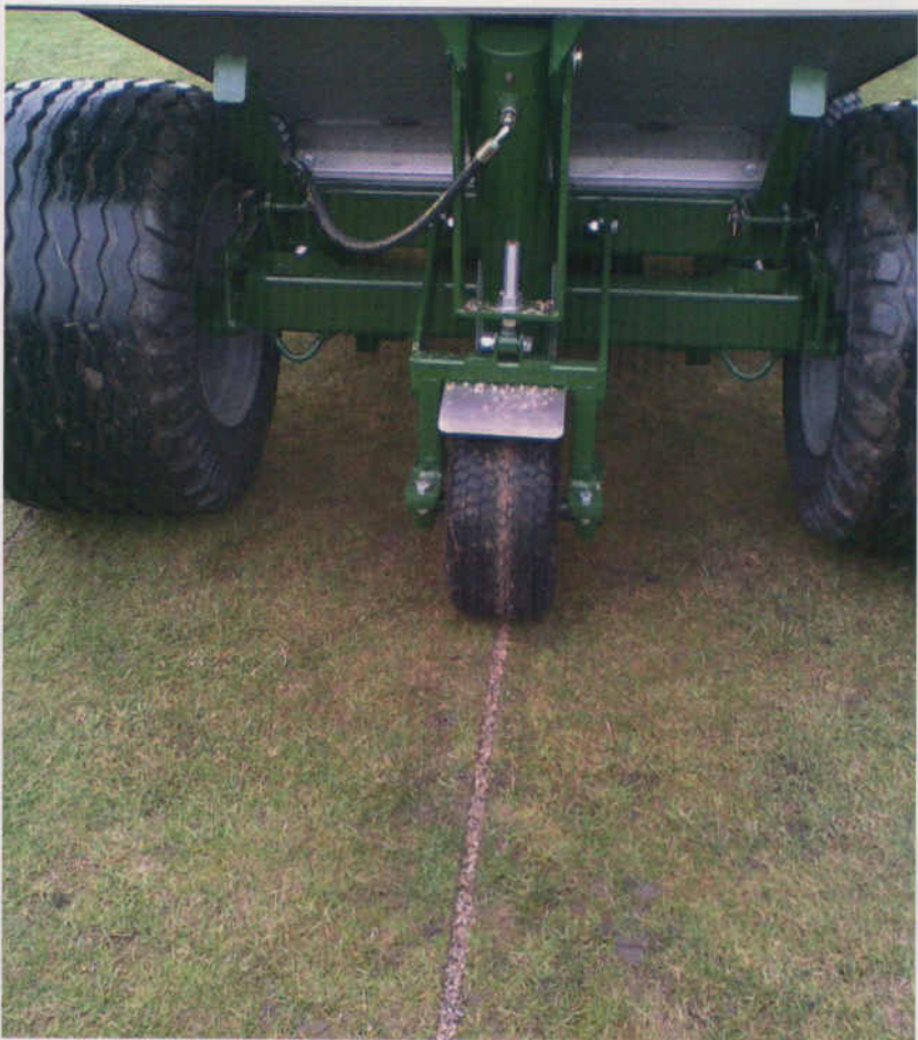
Three-ton Gravel Band Drainer installing gravel to surface. Aggregate can also be set down in the trench.
