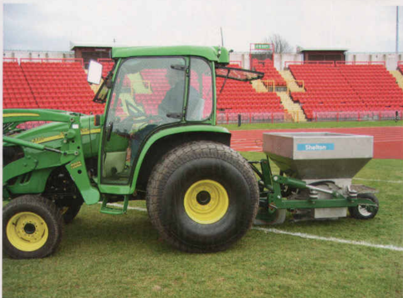
Above: Gravel Band Drainer installing 1-inch wide bands in Gateshead Stadium, England.
