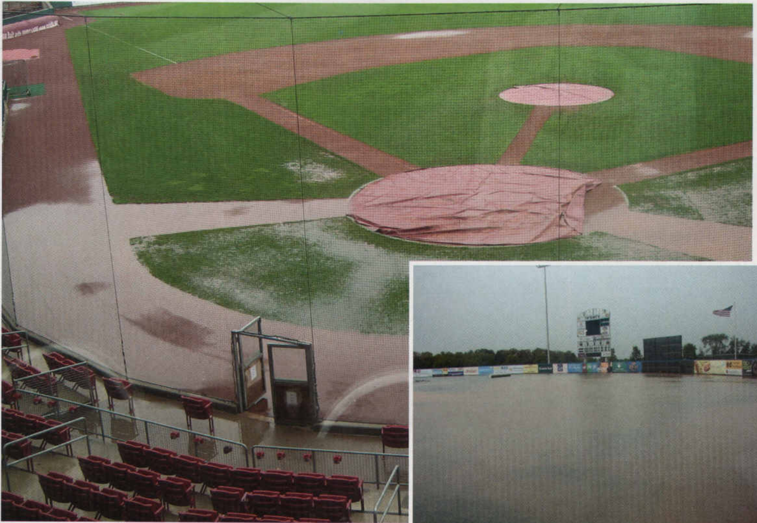
This installed drainage system failed.
