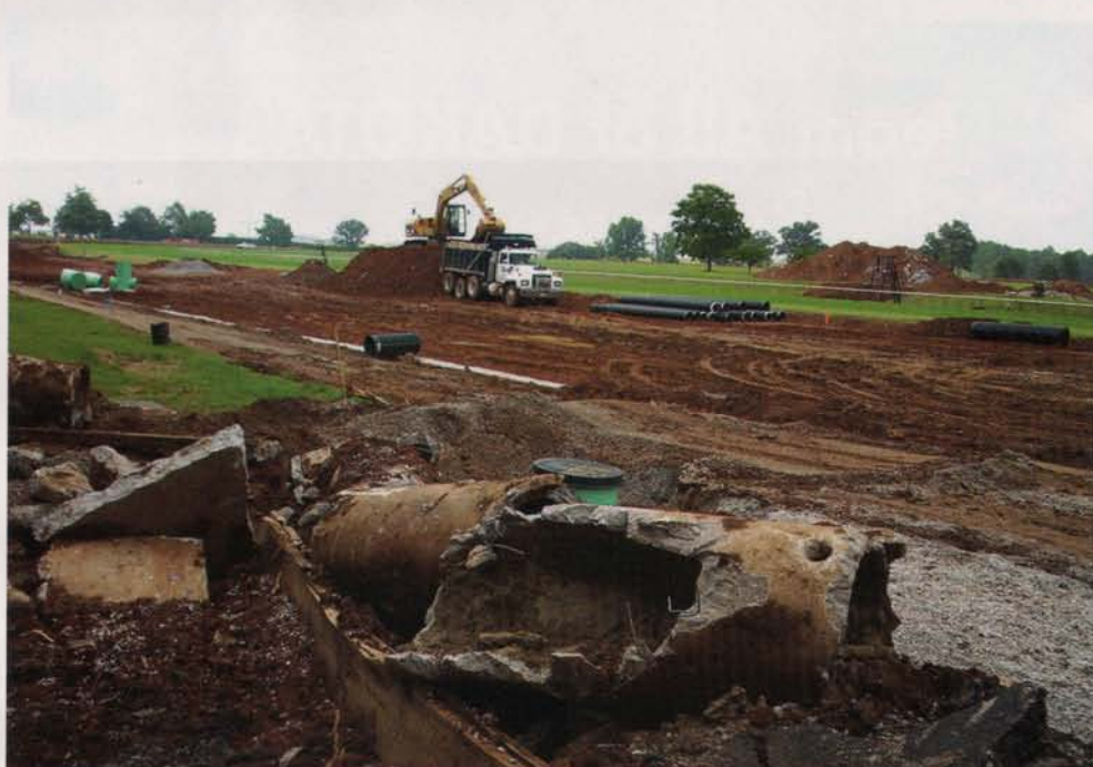
Three runs of perforated pipe were put in, running parallel to each other around the track, spaced 20 feet apart.
