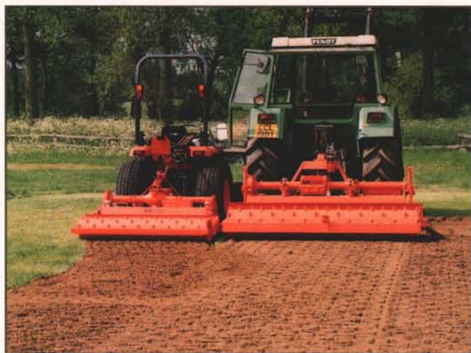
The Net-Avator Soil Conditioner can bury stones to an eight to 10-inch depth, while performing six other ground preparation operations in the same pass.
