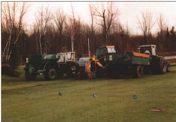
Modern slit drainage equipment limits installation time even in existing fields by simultaneously cutting, excavating, and filling slits in one pass. Courtesy: Lanco.
