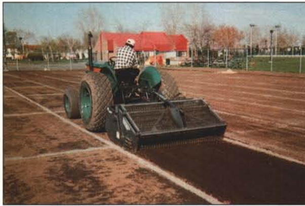
Installing modern slit drainage in new field constructions is a very straight-forward and quick process. Courtesy: Lanco.
