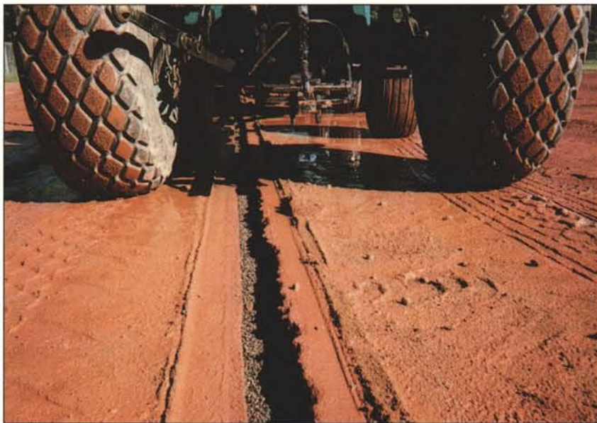
A typical slit drainage installation consists of a series of narrow trenches cut into the playing surface and filled with a drainage medium, such as pea gravel, fine crushed stone or coarse drainage sand. Courtesy: Lanco.
