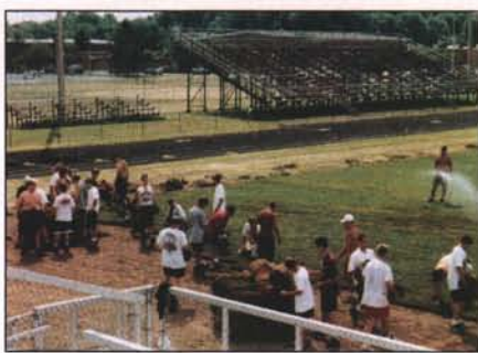
This football field reconstruction project was completed at about half the usual price because of community participation. Volunteers included members of the football team, who turned out to help lay the sod they would play on. Courtesy: Jim Puhalla
