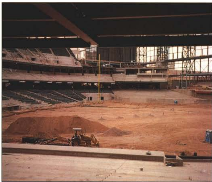
Shown during its construction, BOB is a probable Seminar on Wheels stop for the STMA's 1999 Conference. Courtesy: Trusty & Assoc.
