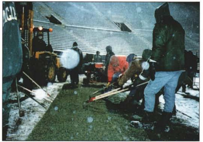
Finishing up the job in a driving snow storm, workers move a tarp in as the last strip of sod is pulled up and rolled.
