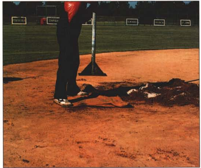
French Drain — Step Four. Tamp approximately two inches of loose clay over the opening for consistent and even playing surfaces.
