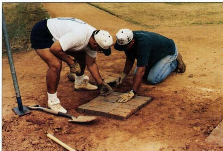
Renovating a diamond, Dave Ashman (left) and Chris Bunnell install unfired clay bricks on both sides of home plate to strengthen one of the most heavily used areas.
