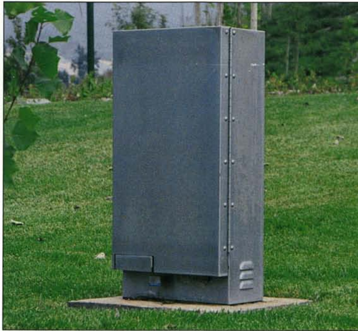
A stainless-steel enclosure protects a controller and delicate circuitry in a park setting.
