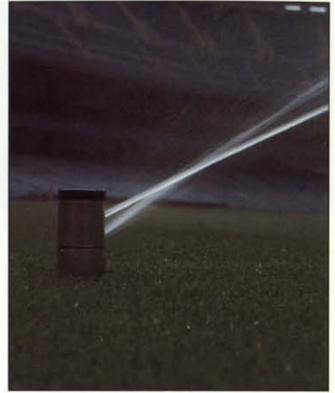
Irrigation systems should be winterized before the first freeze. Photo courtesy: Rain Bird.
