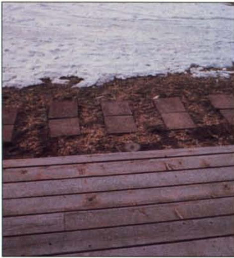
Any system in an area with freezing and below freezing temperatures during the winter is susceptible to damage from the cold. Photo courtesy: The Toro Company-Irrigation Division.
