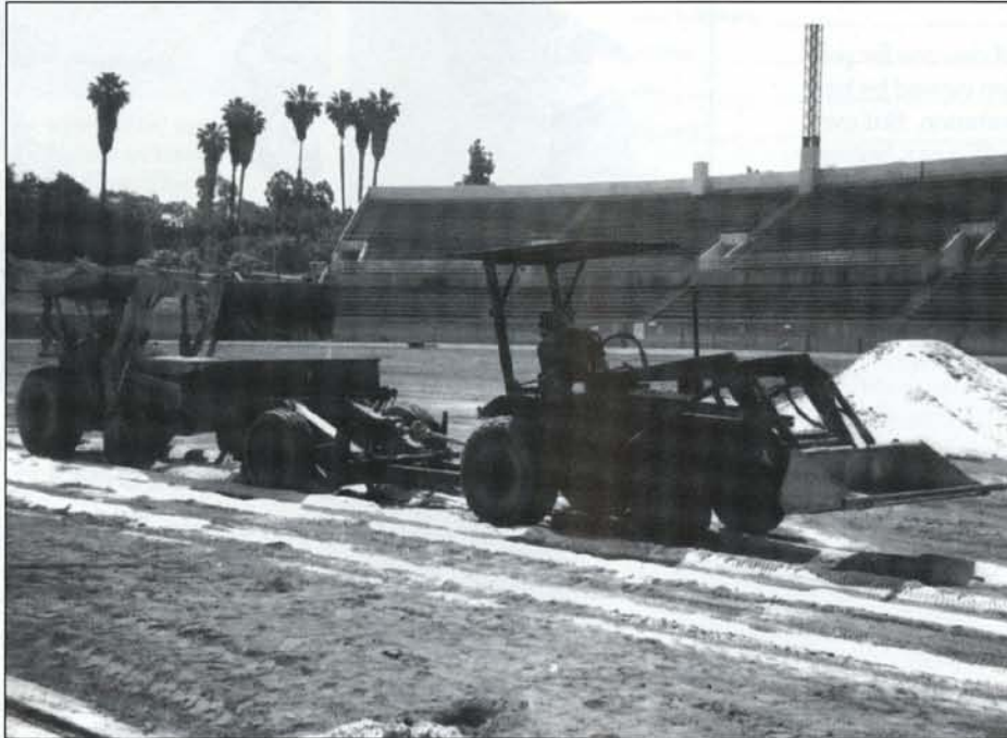
Subsurface drainage, installed during field construction or retrofitted, combined with properly designed and constructed soil profile, is the key to turf health, as well as most water “ponding” problems.
