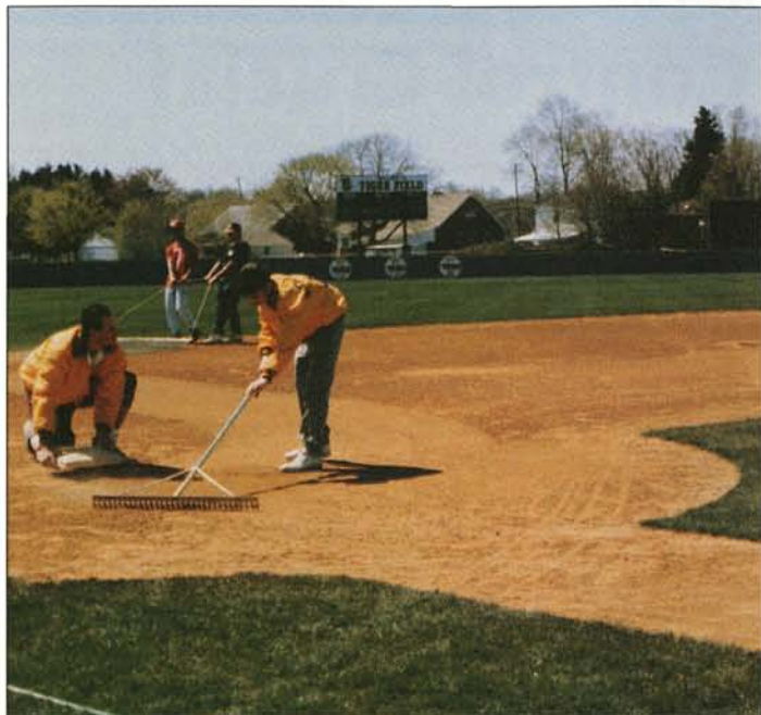
To repair holes, add premoistened packing clay and use a hand-held tamping device to work the packing material firmly into place.
