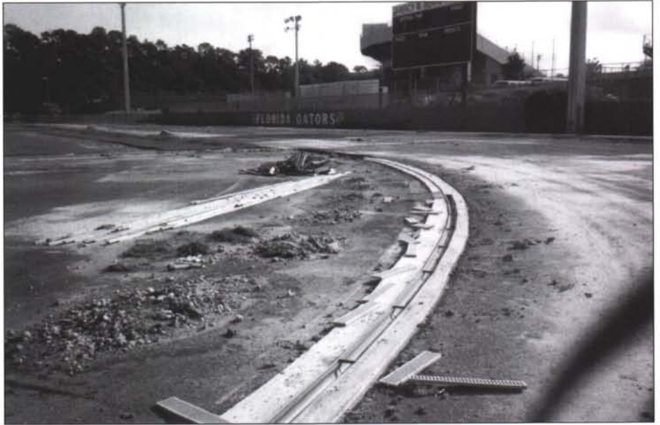
Perimeter catch basin at the University of Florida. Photo courtesy: NDS.
